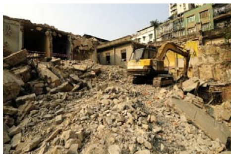
Demolition works at Rua da Penha mark the start of its redevelopment programme.
