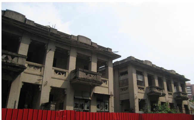
Demolition works at Rua da Penha mark the start of its redevelopment programme.
